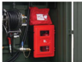
Spill kits & fire extinguisher
