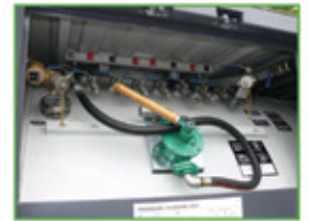
Control hatch of TCT series tanks shown
